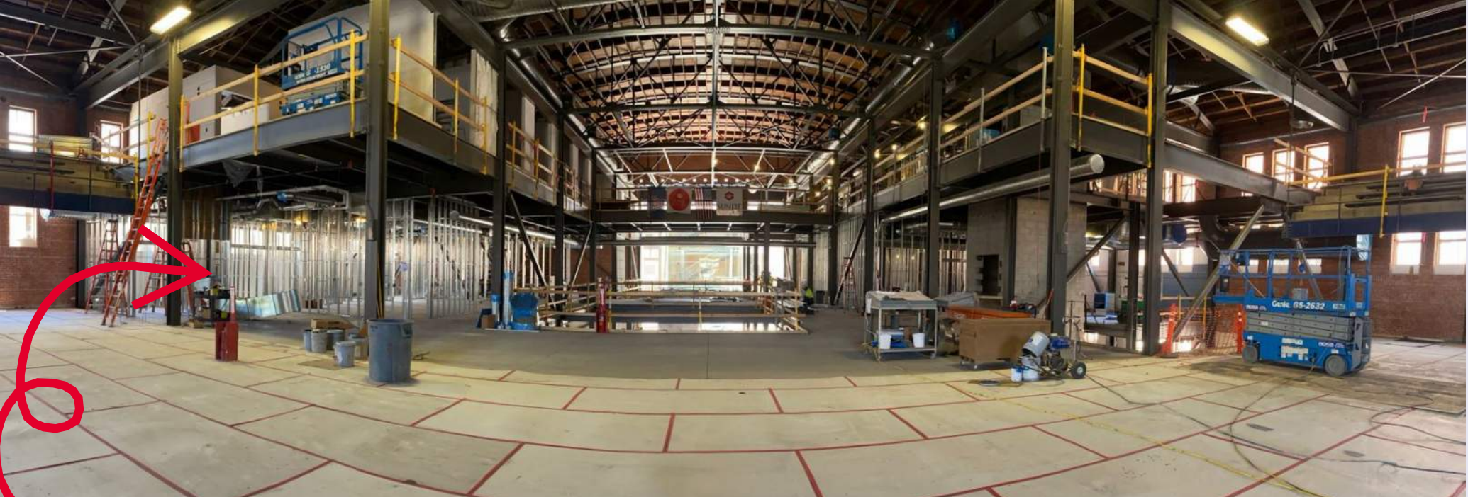
Inside the main entrance standing on the historic gym floor, looking south. Level 3 drywall and level 2 framing are underway. Mechanical, electrical, plumbing, and fire sprinkler systems rough-in are commencing on all three levels!
